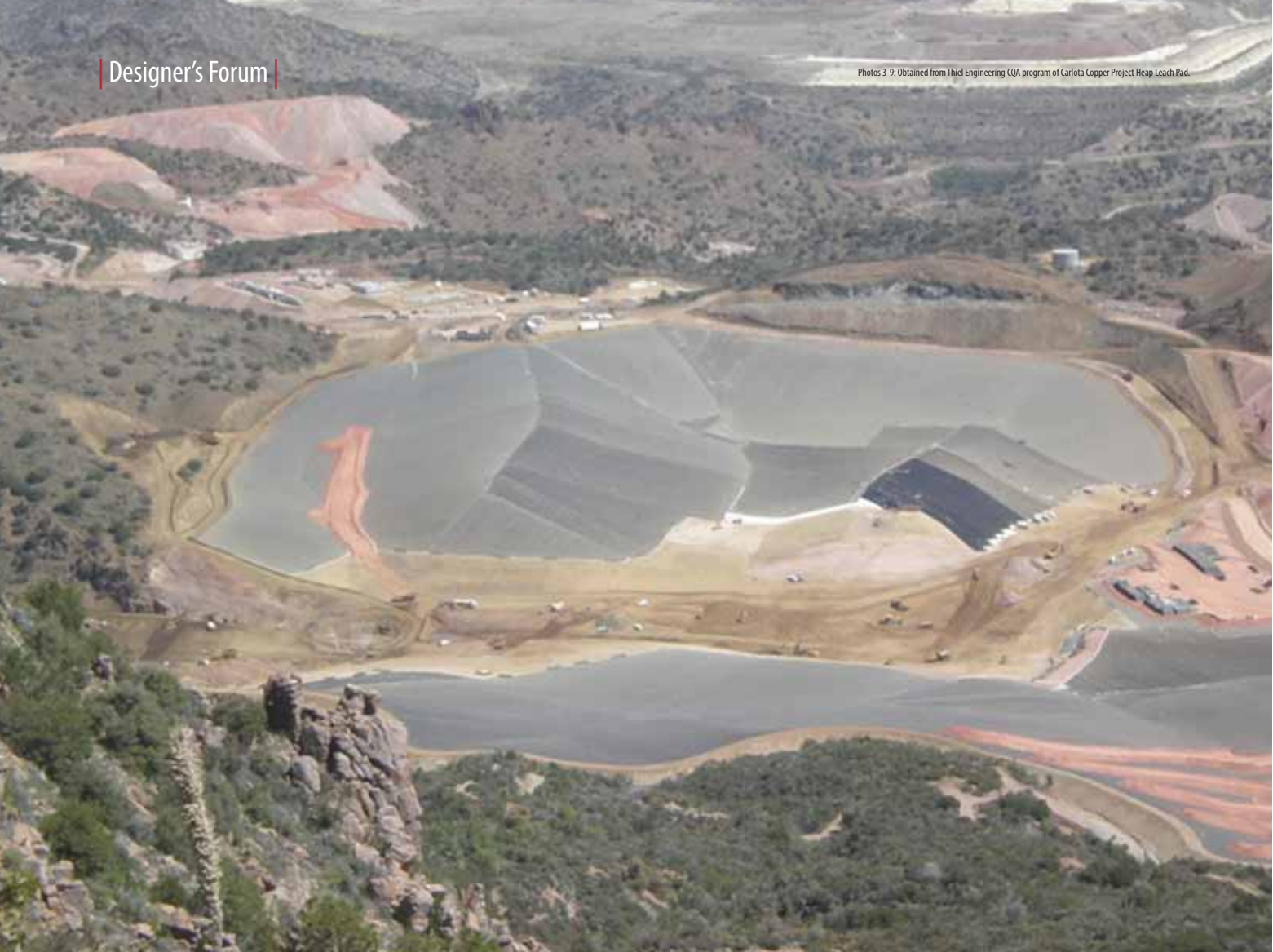
Figure 3 | The Carlota Mine heap leach pad under construction with approximately 150 acres of GCL/geomembrane composite liner.
