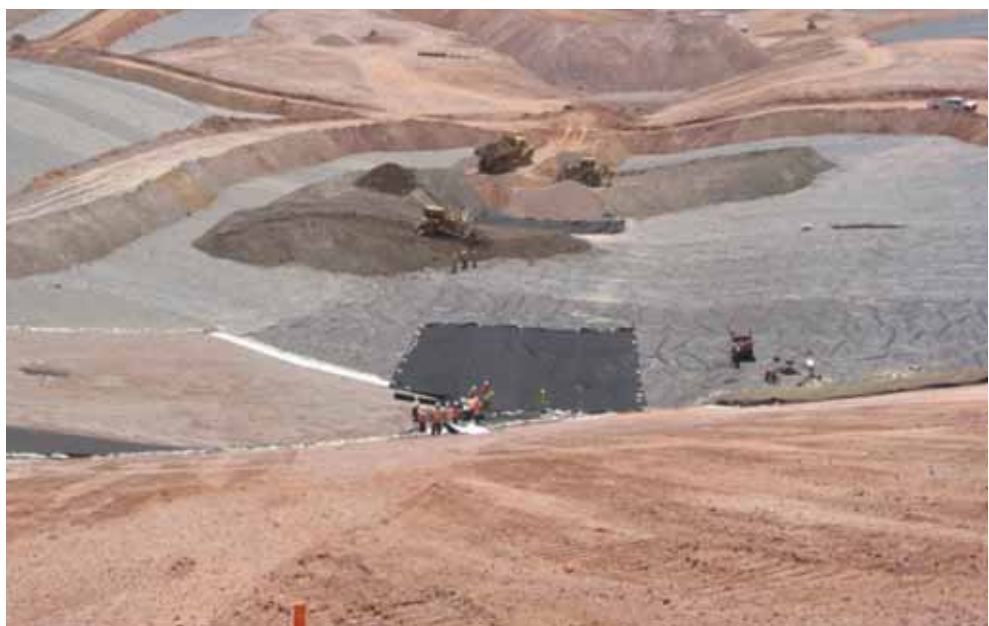
Figure 6 | Some areas of liner that were unballasted and some areas covered with overliner material.
