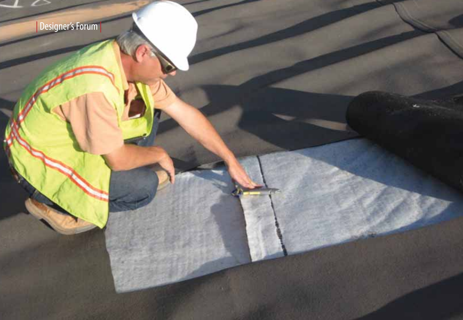
Figure 7 | Exhumation of GCL overlap on slope that had been unballasted for more than 60 days. The heat-tacked seam was intact.
