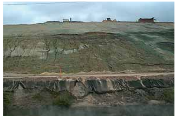
Photo 1. Slumps and erosion rill on a 2H:1V slope of a paper mill sludge landfill. From Richardson et al. (2004).
