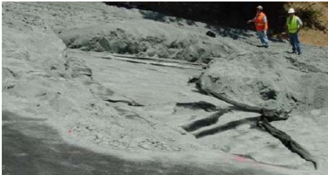
Figure 3. Geocomposite internal failure on 2:1 slope (Exposed surface in center of photo is the delaminated geonet core).
